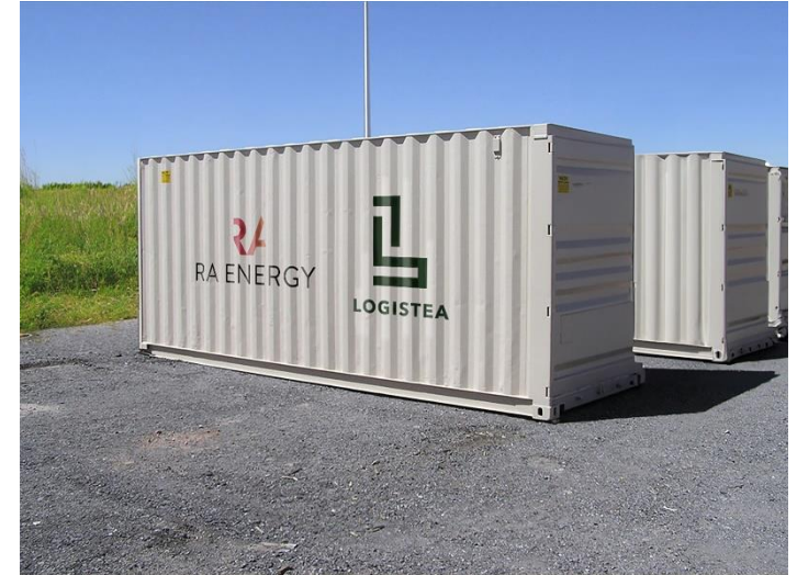
Illustration Vaggeryd Logistikpark battery park
