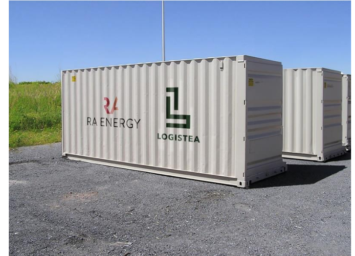
Illustration Vaggeryd Logistikpark battery park
